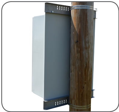
Enclosure is fastened to the pole with 4 clamps and two brackets
